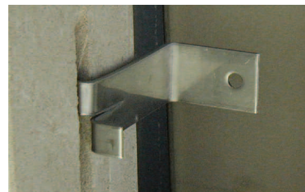
Photo A. Head joint anchors miss 90% of metal stud area
