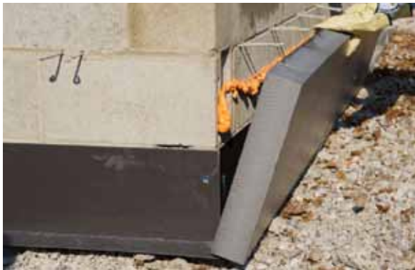
STYROFOAM™ Brand CAVITYMATE™ Ultra Insulation Boards are secured between wall ties with GREAT STUFF PRO™ Gaps & Cracks Insulating Foam Sealant, which also acts as an air/vapor barrier between board edges.
